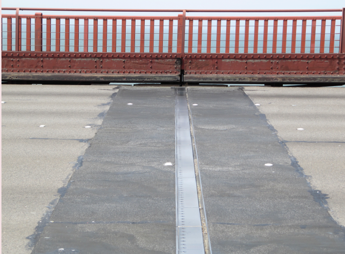
Expansion joint on the Golden Gate Bridge. Image Credit: Expansion Joint Golden Gate Bridge by Michiel1972 via Wikimedia Commons
