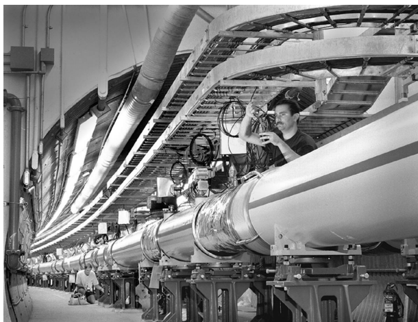
FIGURE 6 Inside the tunnel of the relativistic heavy ion collider (RHIC) during installation work. [Courtesy of BNL.]
