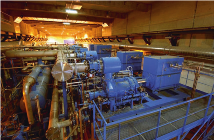
Fig. 2.21 Image of compressor station at CERN
