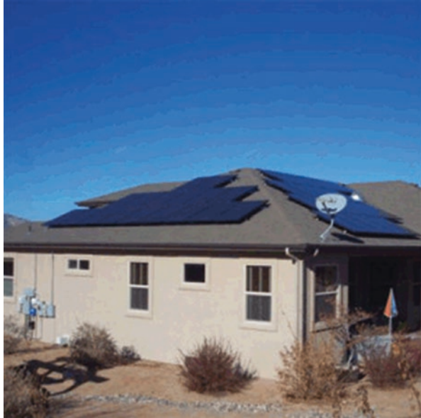
Fig. 1.4 A house with a solar system
