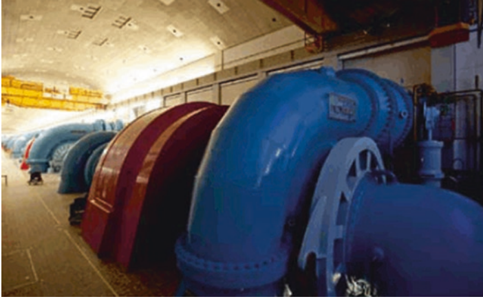
Fig. 1.9 Turbine hall of the Vianden pumped-storage power plant (Courtesy of RWE of German Power Company)
