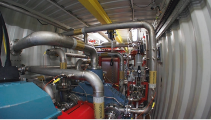
Fig. 3.5 All the component parts involved in the CES chain (Courtesy of Highview Power Storage)
