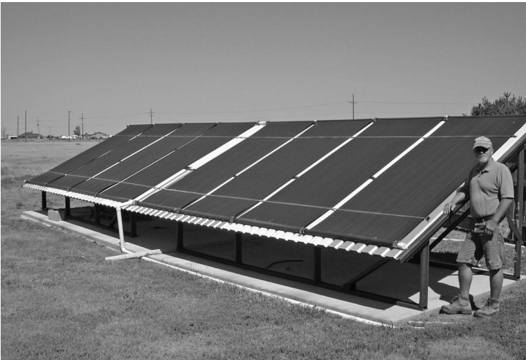
FIGURE 5.20 Solar hot water system for heating a swimming pool. Fixed tilt angle of array is 27^\circ for summer sun at 35^\circ N. Eight panels, thermoplastic, each 1.2 by 3 m (4 by 10 ft).
