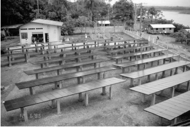
FIGURE 6.17 A 50-kW PV array with controller and a large battery bank were added to the diesel station in the village of Campinas, Amazonas, Brazil. (From National Center for Photovoltaics, National Renewable Energy Laboratory (NREL), www.nrel.gov/ncpv .)
