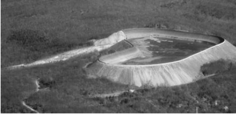
FIGURE 13.8 Upper reservoir for Taum Sauk pumped hydro plant, Missouri. Notice scouring of the creek due to wall failure. (Source: U.S. Geological Survey photo 037.)
