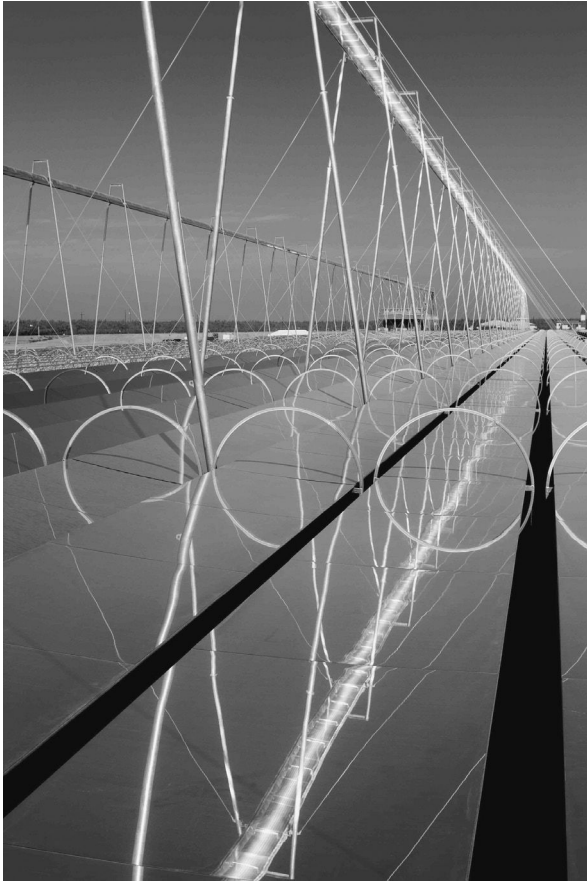
FIGURE 7.11 Close-up of mirrors (each 2 m wide) and receiver tube, which is 18 m above ground, Kimberlina plant. (From Sandia Labs.)
