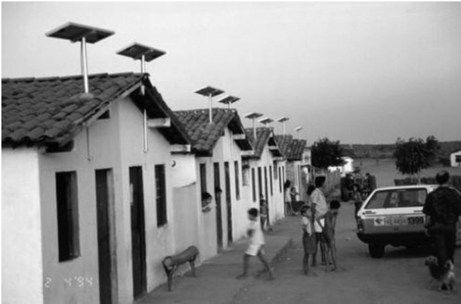
FIGURE 6.19 PV systems (50 W) for two fluorescent lights, village of Cacimbas in the state of Ceara, Brazil. Notice the tilt angle of the collectors. (From National Center for Photovoltaics, National Renewable Energy Laboratory (NREL), http://www.nrel.gov/ncpv .)
