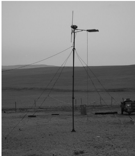
FIGURE 9.16 Small wind turbine, 50 W, isolated household, Inner Mongolia, China. Notice rope on tail for manual control; however, this control mechanism is not recommended by manufacturer.
