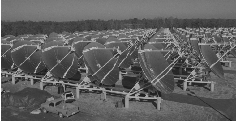
FIGURE 7.15 Solar Total Energy System, 144 dishes, 7 m diameter, at textile plant near Shenandoah, Georgia. The dishes provided thermal energy for process heat and air conditioning at a nearby textile mill. (From National Center for Photovoltaics, NREL, http://www.nrel.gov/ncpv .)
