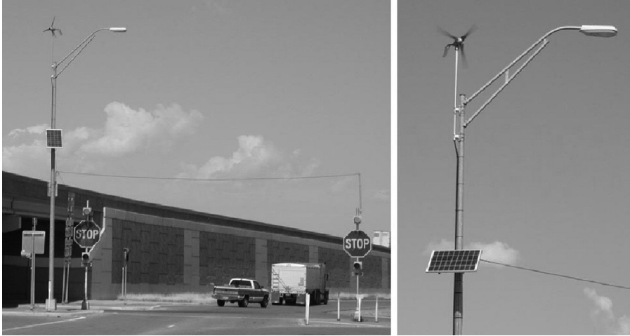
FIGURE 9.20 PV-wind powers streetlight and flashing red lights at stop signs, McCormick Road on I27 between Canyon and Amarillo, Texas.
