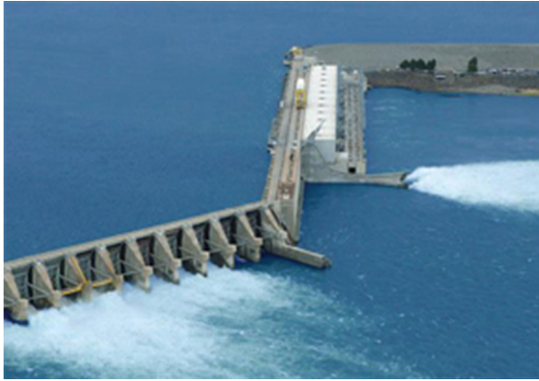
Figure 2.1. Hydroelectric facility. ( Source: Photo courtesy of National Renewable Energy Laboratories (NREL).)
