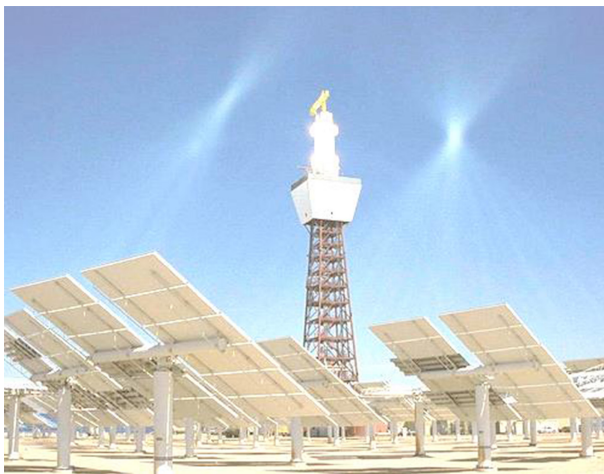
Figure 8.7. Solar thermal plant.
