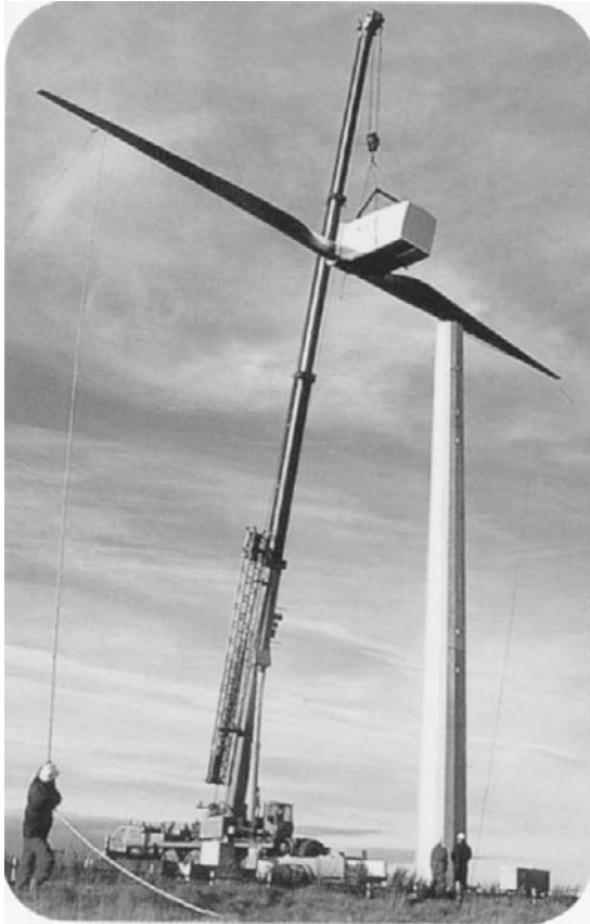
FIGURE 4.6 WEG MS-2 wind turbine installation at Myers Hill. (From Wind Energy Group, a Taylor Woodrow subsidiary and ETSU/DTI, U.K.)
