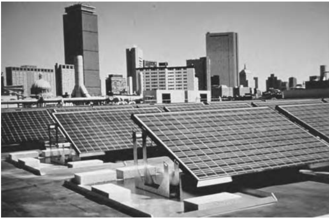
FIGURE 13.2 18 kW grid-connected PV system on the Northeastern University Student Center in Boston. (Source: ASE Americas, Billerica, MA. With permission.)
