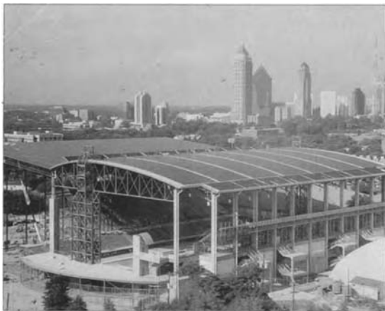
FIGURE 8.8 Roof of Atlanta’s Aquatic Center with 345-kW grid-connected PV power system. (From Georgia Institute of Technology. With permission.)
