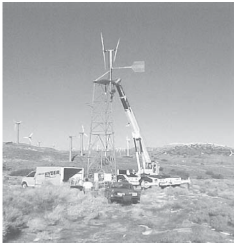
FIGURE 19.19 Contrarotating turbine installation on a 50-ft tower at Oak Creek Energy Systems test site in Mojave, CA.
