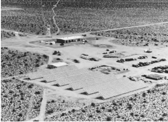
FIGURE 12.6 A 300-kW PV–diesel hybrid system in Superior Valley, California. (From ASE Americas, Inc., Billerica, MA. With permission.)
